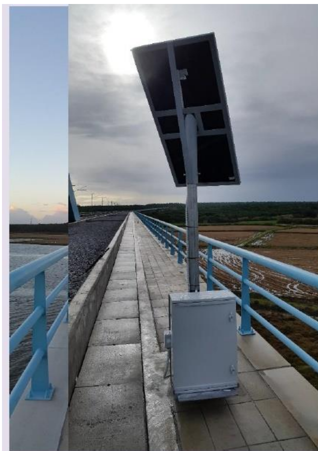
FIGURE 9. LOCATION OF THE MAIN LOCAL STATION A) AND ILLUSTRATION OF INSTALLATION B)
