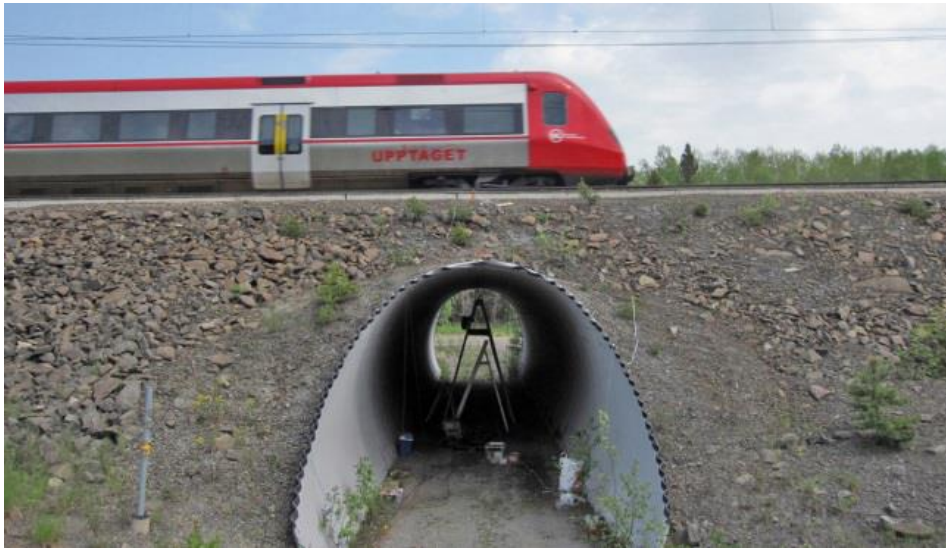
FIGURE 40. THE SOIL-STEEL COMPOSITE BRIDGE AT MÄRSTA DURING PASSAGE OF AN X52 TRAIN, REPRODUCED FROM
