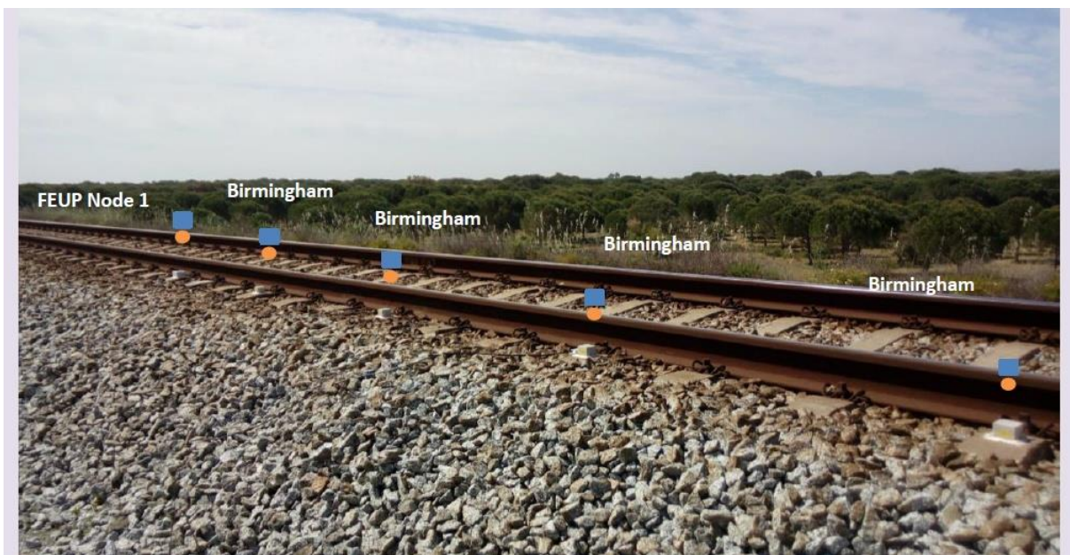
FIGURE 17. SENSORS DISTRIBUTED IN THE TRANSITION
