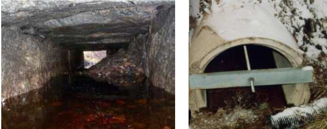
Figure 4.2.32. Left: Old stone culvert where the boulders have separated and sand and mud have poured down. Right: A culvert is kept together by post-tensioning of steel bars Sjöberg et al (1998), TRVH Avvattning (2011).
