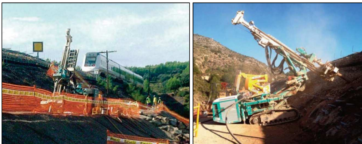
Figure 4.1.27. Execution of injections at the side of the in-service track (Lopez Moreno, 2013)
