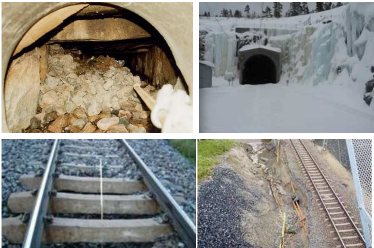
Figure 4.2.30. Examples of damages in culverts (from top left clockwise): (a) Cracking and downfall of bank material; (b) Ice clogging the culvert; (c) Crater in bank due to downfall of material into culvert; (d) Erosion along bank. TRVH Avvattning (2011).
