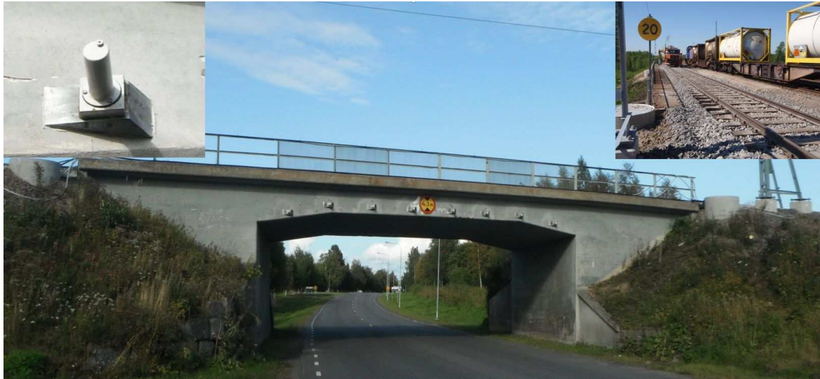
Figure 4.2.16. An upgraded concrete trough bridge built in 1959 in Haparanda in northern Sweden. In 2012 the bridge was strengthened with eight post-stressed bars installed in holes drilled through the slab (insert left). In this WAY, it was possible to increase the bending and shear capacity of the slab to enable an upgrading of the line from an axle load of 25 to 30 tonnes. ML-D1.1 (2013), Nilimaa et al (2013, 2014, 2015).
