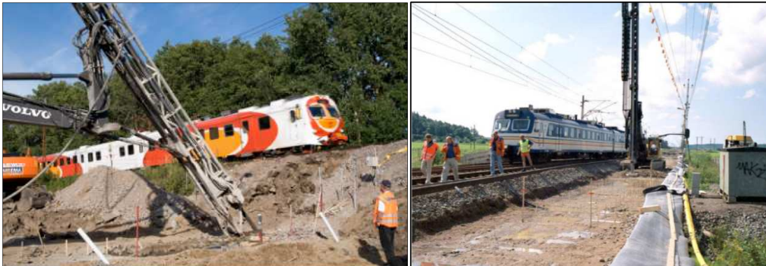
Figure 4.1.17 Example of installation of a lime column. Left: Inclined; Right: Vertical (INNOTRACK, 2008)
