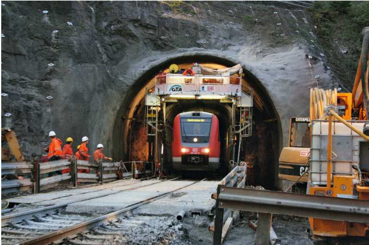
Figure 4.2.25. Jährod Tunnel in Germany being enlarged by the Tunnel-in-Tunnel (TIT) method, Simon (2012).
