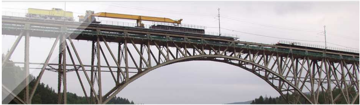
Figure 4.2.6. Top: Forsmo Bridge over Ångerman River, Sweden, after strengthening; Bottom: Steel truss arch with replacement of top structure at the Forsmo Bridge. Collin et al (2010).
