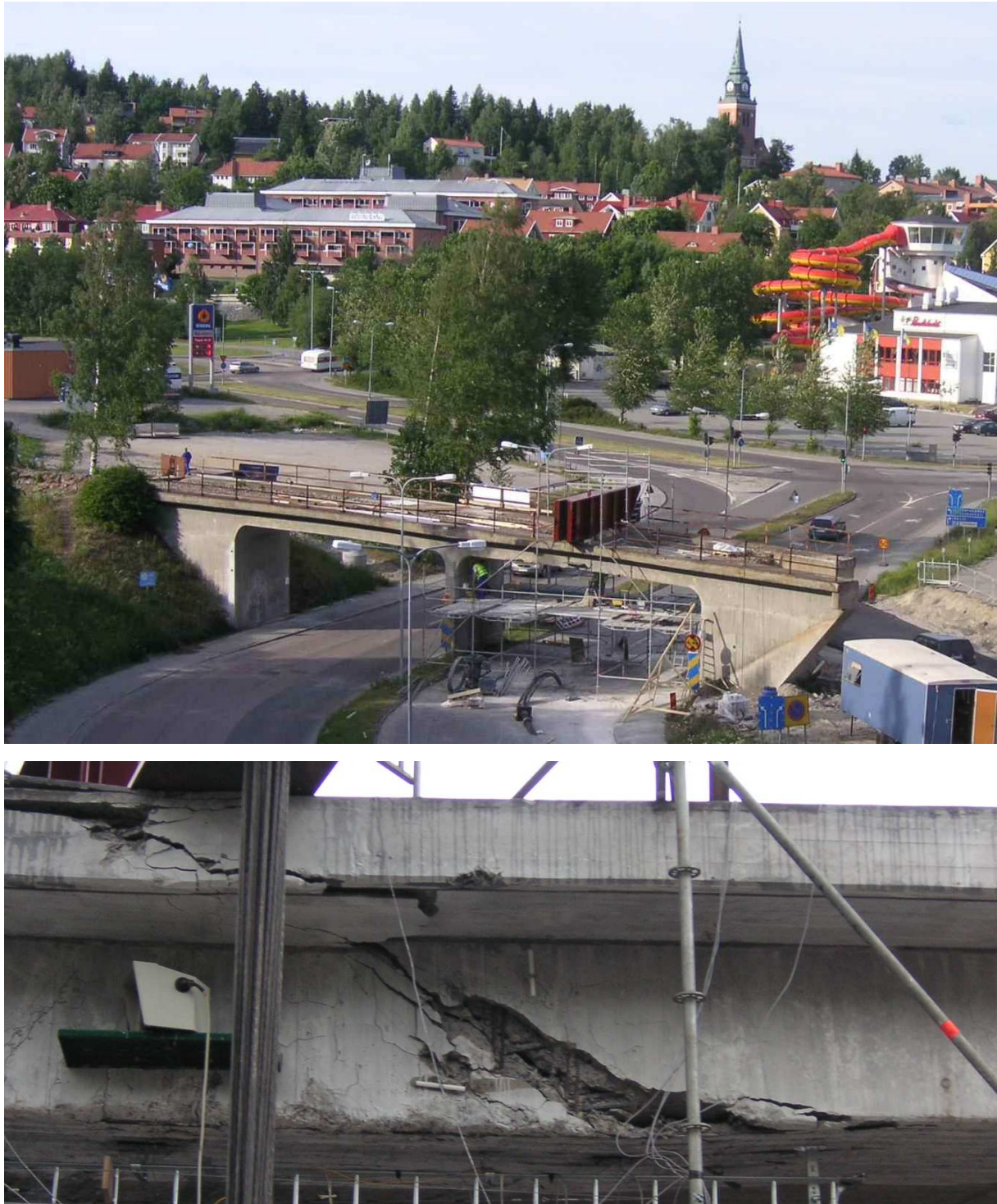
Figure 4.2.20. Test to failure of a strengthened trough in Örnsköldsvik, 2006. Top: Overview of bridge with East rail bank cut away and replaced by a temporary road to substitute the lane under the bridge span being tested. Below: Detail of failure in South beam caused by a combination of stresses due to bond, shear, bending and torsion. SB-D7.1 (2006), Puurula et al (2012, 2013, 2015).
