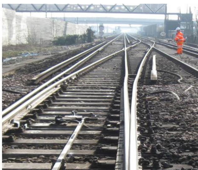
Figure 4.2.2. Misalignment at switch heel due to thermal forces
