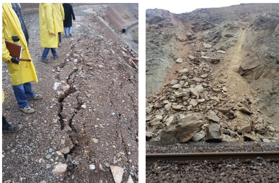
Figure 4.3.4. Landslide due to excessive rain (left) and unavailable track due to fallen rocks caused by excessive rain (right)
