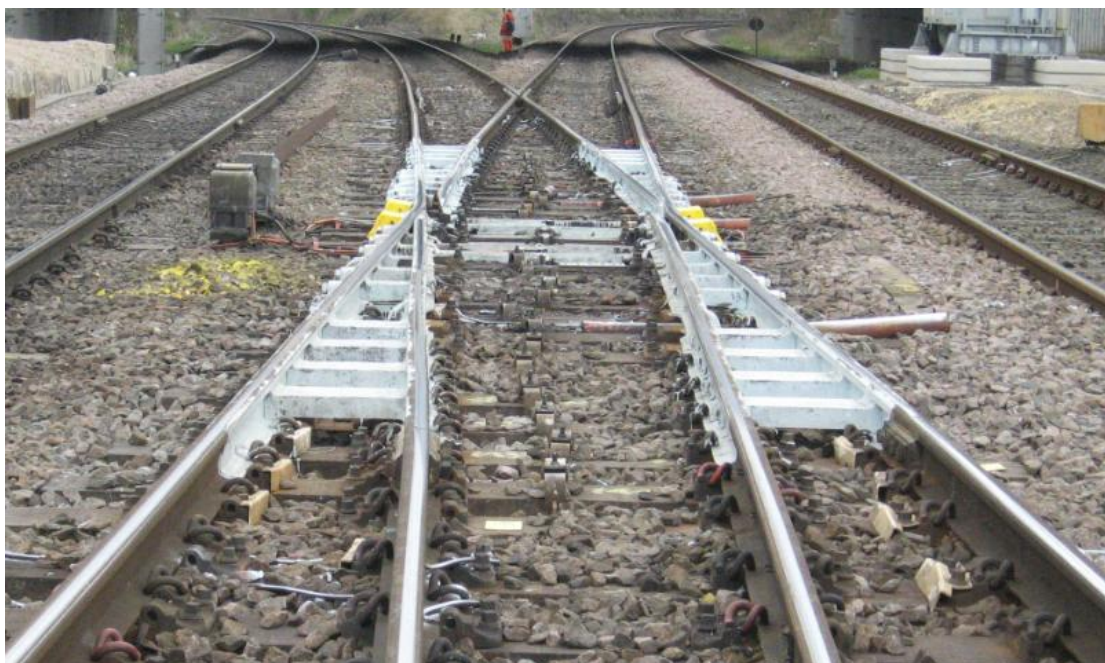
Figure 4.2.3. Switch diamond with heat-reflecting paint
