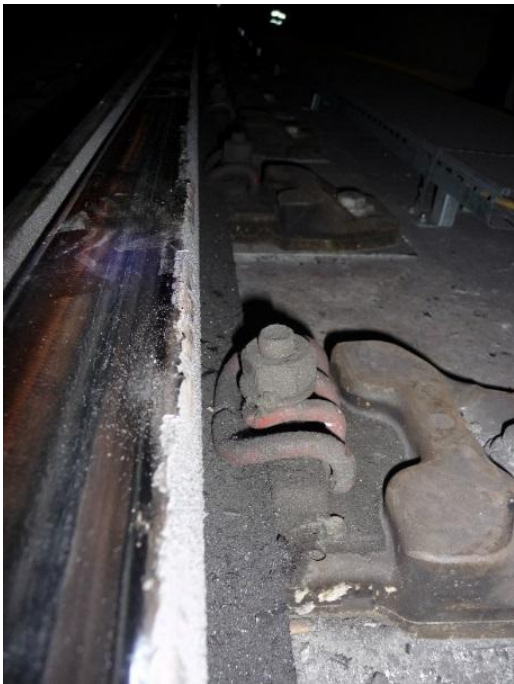
Figure 3.1.5. Stock rail on the right side. View of the field side seen from the switch toe
