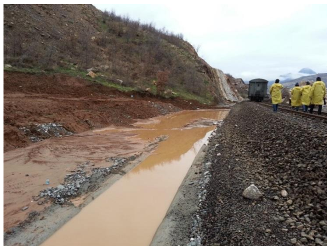
Figure 4.3.2. Drainage failure due to excessive rain
