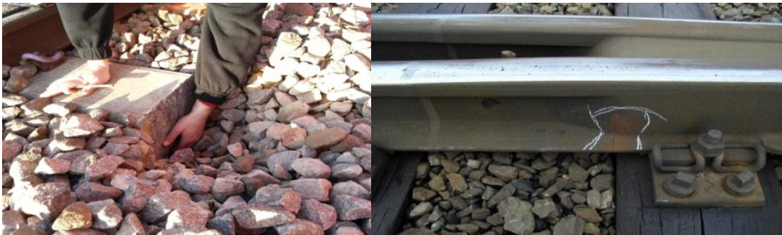
Figure 3.2.6. Illustration of vertical support damage due to the P2 vertical force: voided sleeper (left) and fatigued cast crossing (right) occurring some distance away from the LTA
