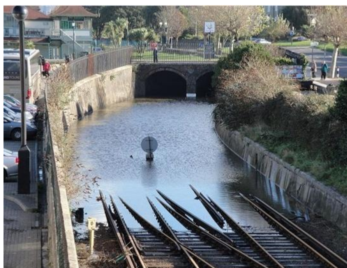
Figure 4.3.5. Flooding in switches and crossings
