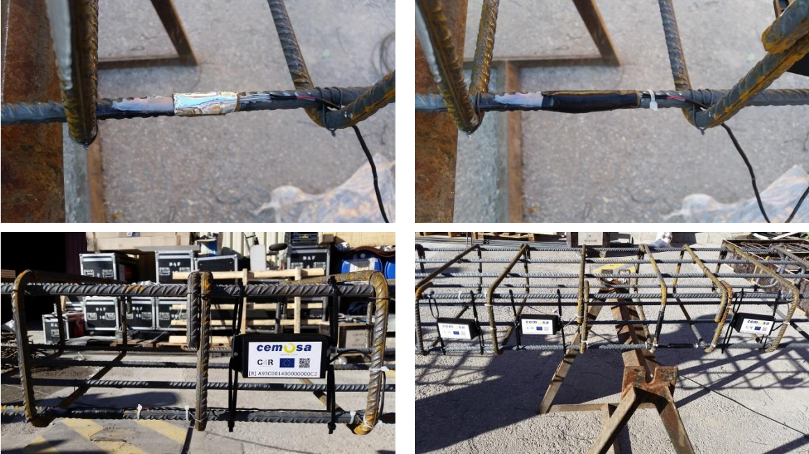
FIGURE 9. PROTECTING STRAIN GAUGE AND INSTALLATION OF RFID V-METER (INSIDE OF PVC BOX)
