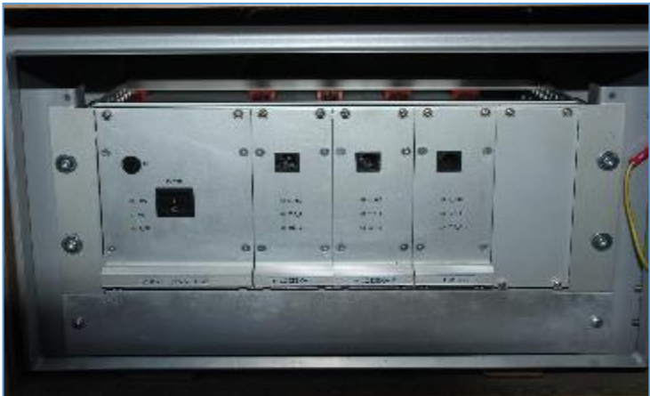
Figure 30 Hot box detector indicator
