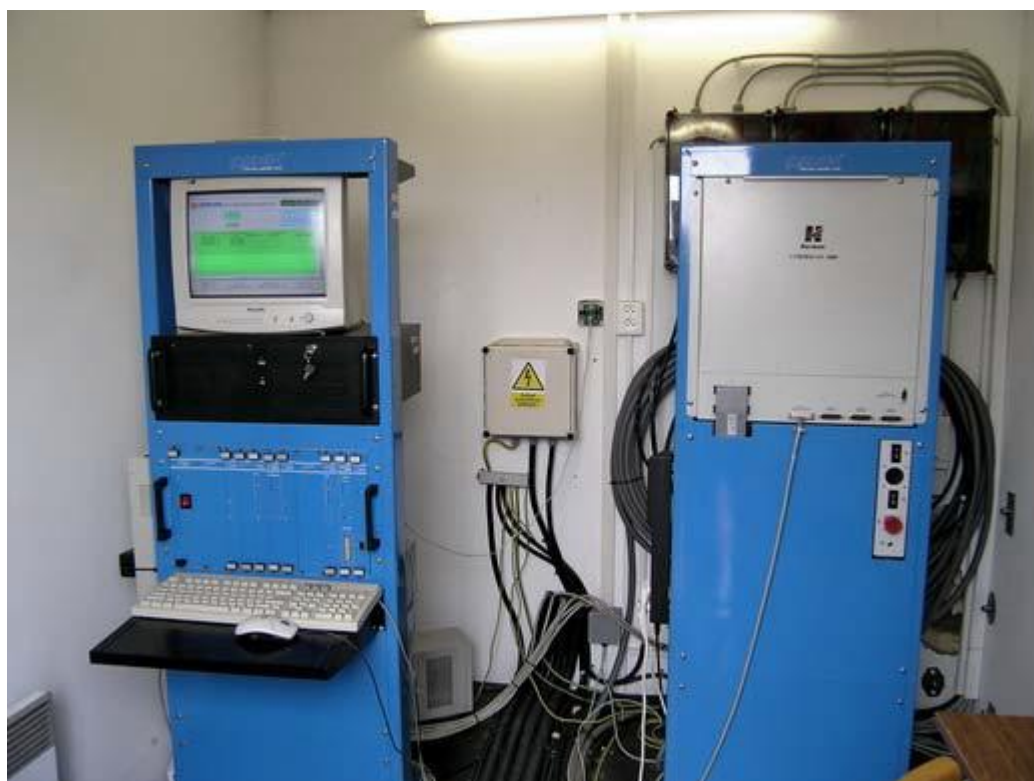
Figure 3 Configuration of the monitoring data equipment
