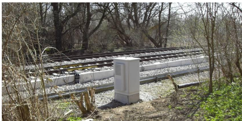
FIGURE 11 MEASUREMENT SYSTEM AND POWER SUPPLY AT THE CRITICAL SECTION
