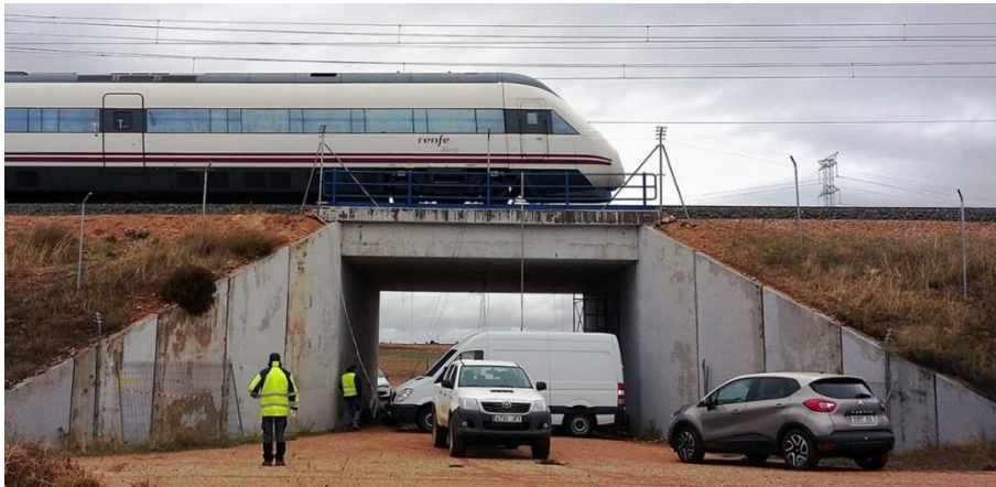
FIGURE 177. Photo of the bridge PI024, during passage of a CAF Alvia S-120 train.
