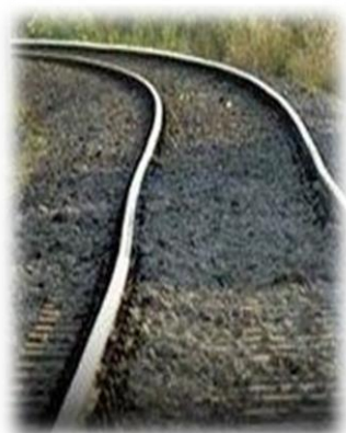
Figure 4.3.1 Failure of track geometry due to warm weather
