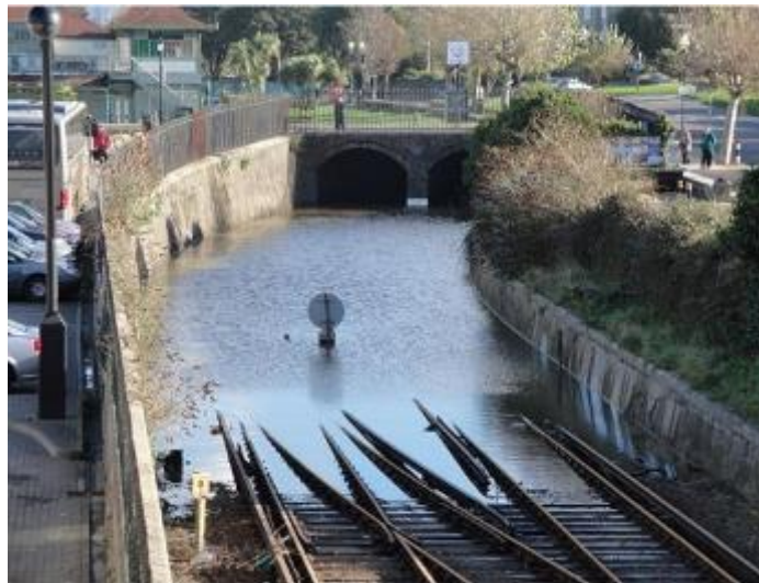
Figure 4.4.5 Flooding in switches and crossings
