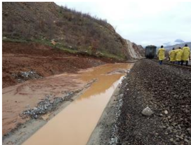
Figure 4.4.2 Drainage failure due to excessive rain
