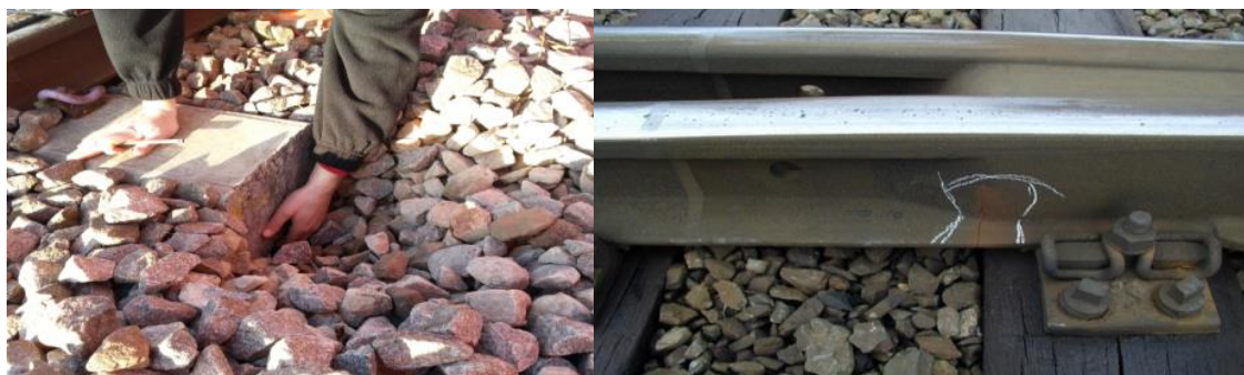
Figure 3.2.6 Illustration of vertical support damage due to the P2 vertical force: voided sleeper (left) and fatigued cast crossing (right) occurring some distance away from the LTA
