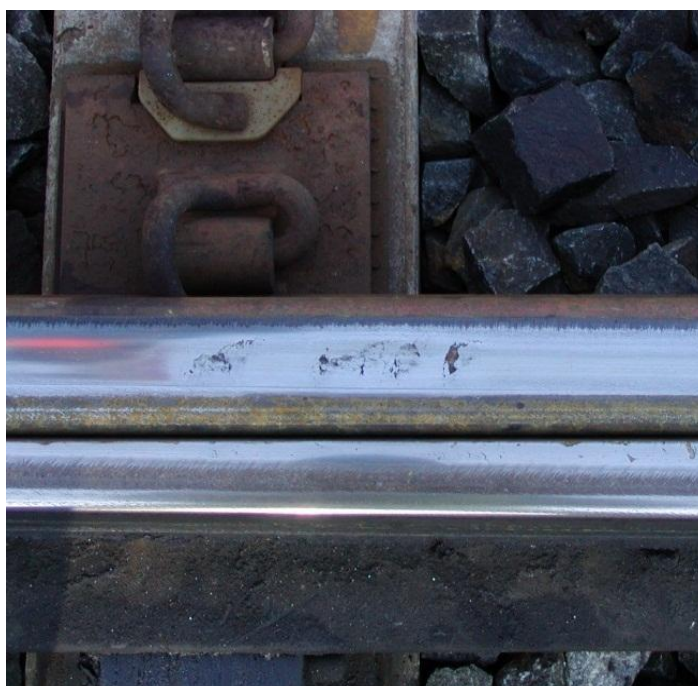
Figure 3.1.1 Wear on the switch rail and RCF on the stock rail caused by high tangential contact stresses. From [3.1.2]
