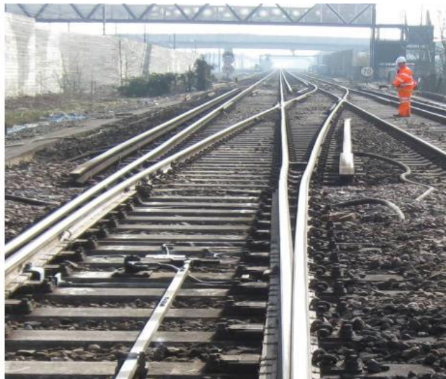
Figure 4.3.2 Misalignment at switch heel due to thermal forces
