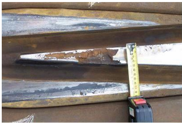
Figure 3.2.53 Spalling Damage in Cast AMS Crossing [3.2.58]
