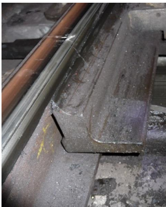
Figure 3.1.3 View of coupled switch rail and stock rail (allowing for diverging track)
