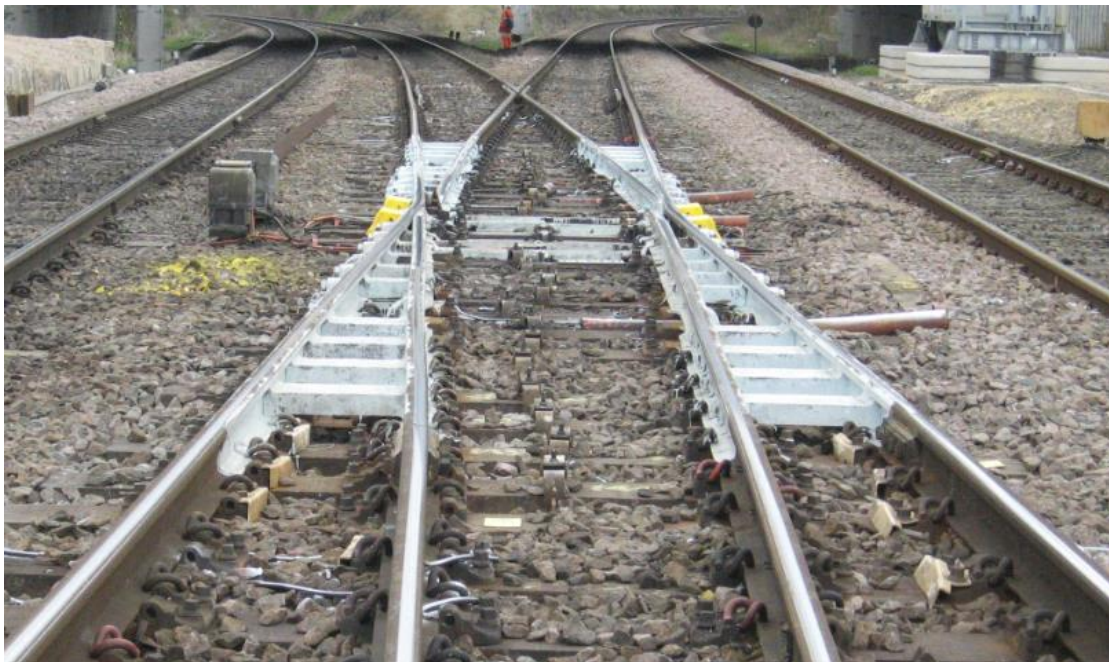
Figure 4.3.3 Switch diamond with heat-reflecting paint
