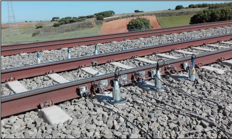
FIGURE 27: SENSORS INSTALLED ON TRACK 1, USED BY THE TRAINS TRAVELLING FROM THE LEFT (MADRID) TO RIGHT (BARCELONA)
