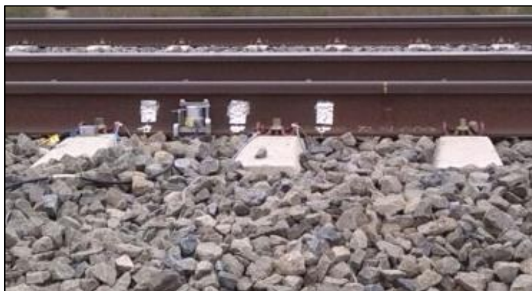
FIGURE 6: PHOTOGRAPH OF THE INSTRUMENTATION INSTALLED IN SLEEPERS T-16 AND T-17: SOME STRAIN GAUGES AND A GEOPHONE IN THE RAIL AND ONE ACCELEROMETER, IN THE LEFT SLEEPER
