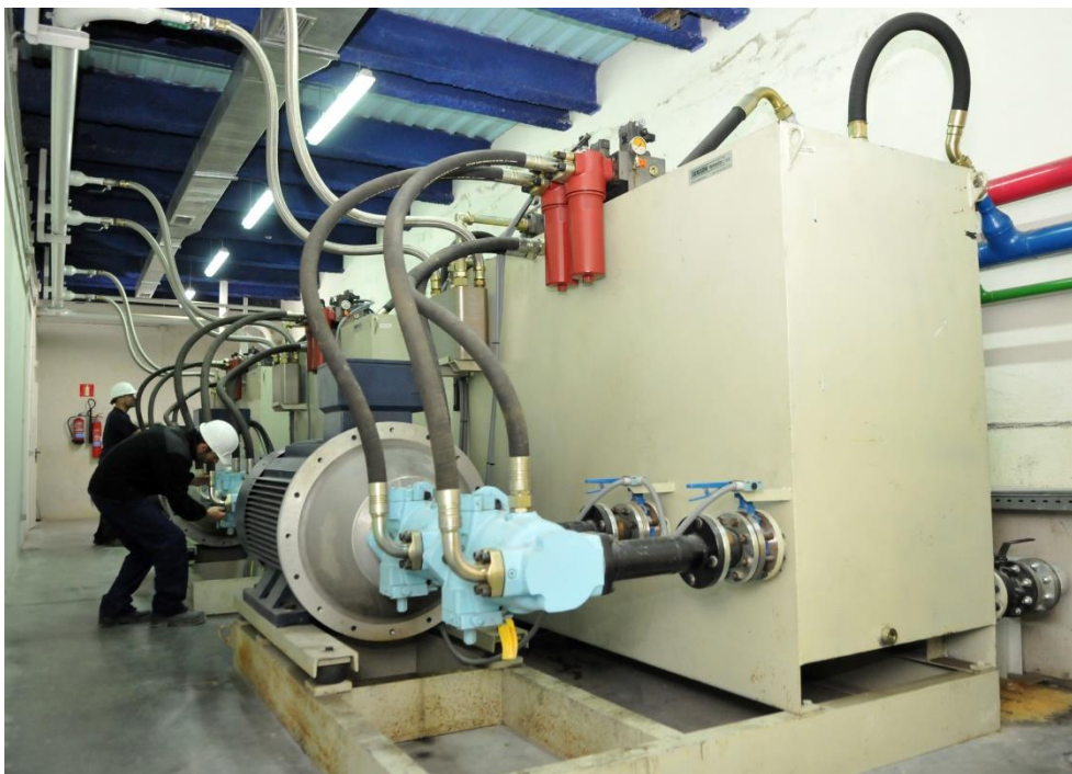
FIGURE 6: VIEW OF THE MOTORS OF THE HYDRAULIC SYSTEM WITH A POWER OF 350 CV EACH TO GENERATE A PRESSURE OF 210 BARS AND A FLOW OF 1800 L/MIN
