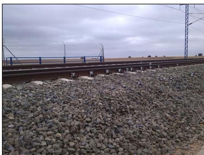
FIGURE 7: PHOTOGRAPH OF THE INSTRUMENTATION BETWEEN SLEEPERS T-5 AND T+7. GEOPHONE SPREAD IN THE RAIL CAN BE OBSERVED
