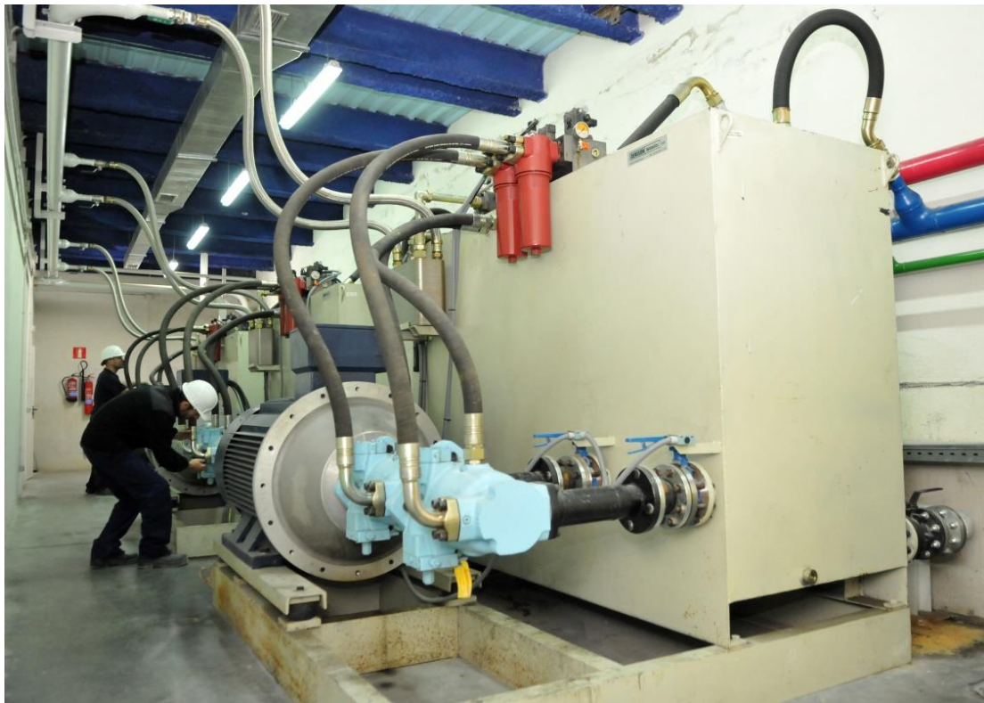
Figure 6: Motors of the hydraulic system with a power of 350 CV each to generate a pressure of 210 bars and a flow of 1800 l/min
